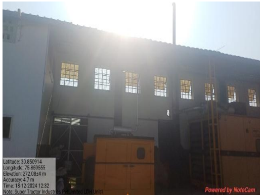
View of DG set 365 KVA and 85 KVA stacks
